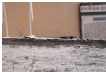
b) Vertical cracks along the middle third of beam
